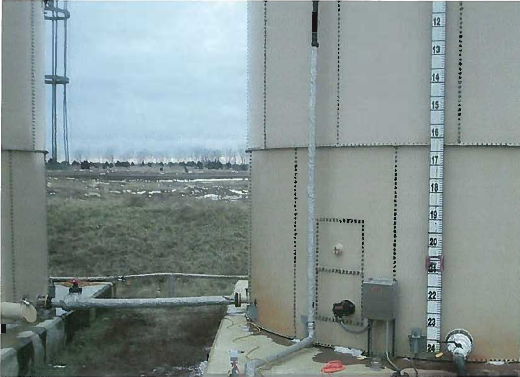
Date: 01/14/2010 Time: 3:22 p.m. Direction: West Photo by: R. Tracy Exposure #: 001 Comments: leachate tank level indicator
