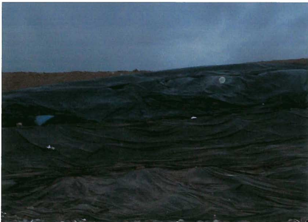
Date: 01/14/2010 Time: 4:53 p.m. Direction: Northwest Photo by: R. Tracy Exposure #: 008 Comments: active area partially covered with tarps
